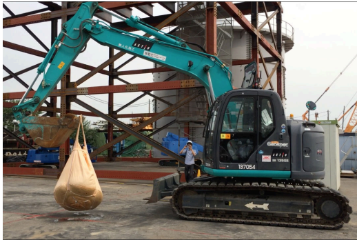
Figure 8: Picking up a Sand Sack and Placing on a Crosshair marked on tarmac
